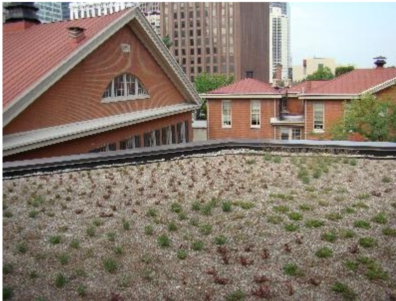
Green roof atop Friends Center, 15th and Cherry, completed May 2007. Source: http://friendscentercorp.org/
