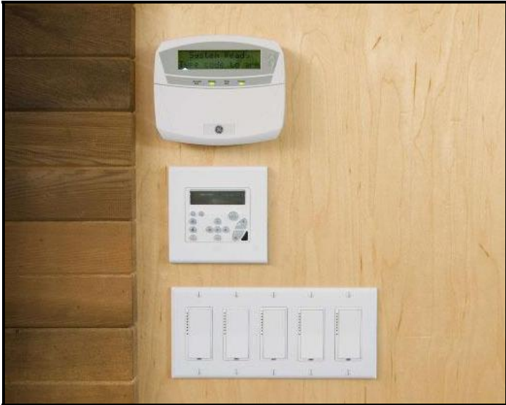
Figure 7. Photo of Home Automation System to Control Lighting and Other Features. Source: www.livinghomes.net
