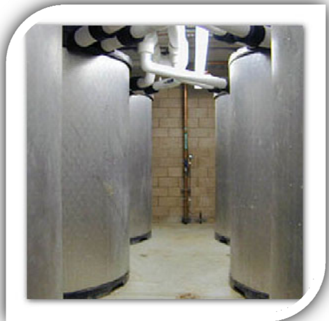
The six ice tanks cool the building during warmer days.
